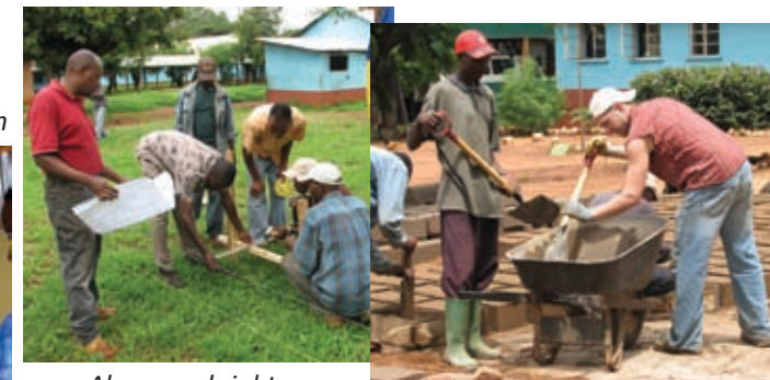
Above and right: Laying the foundation and making concrete blocks for the Infectious Ward Building at Iambi Hospital
